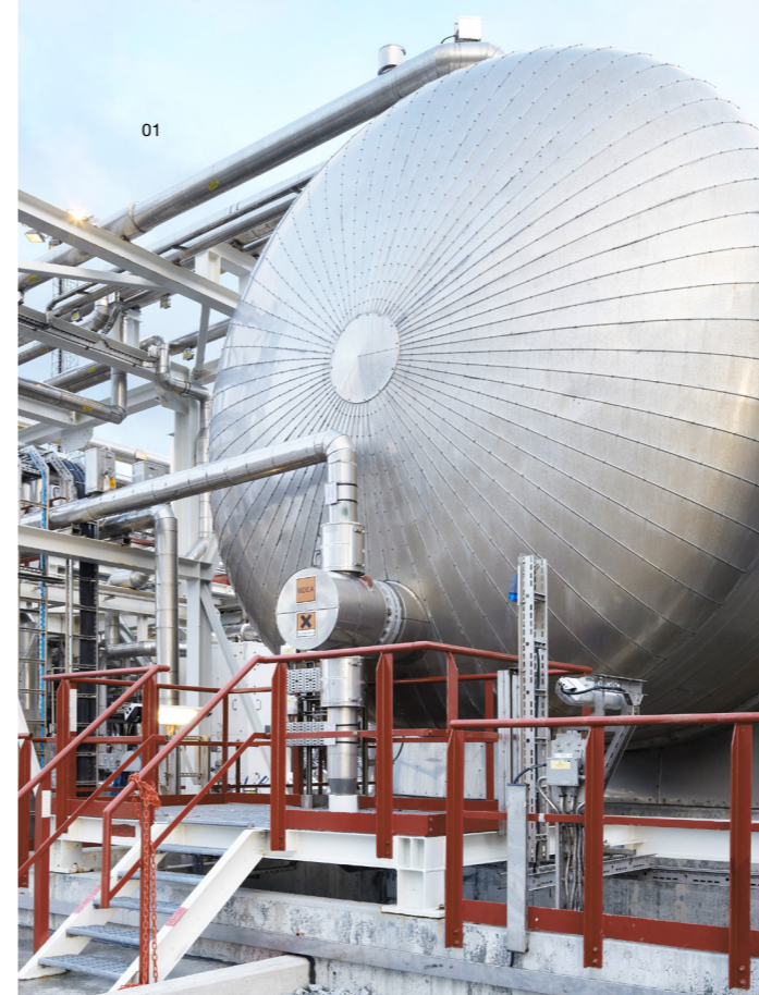
01 Statoil LNG, Melkoya, Norway
